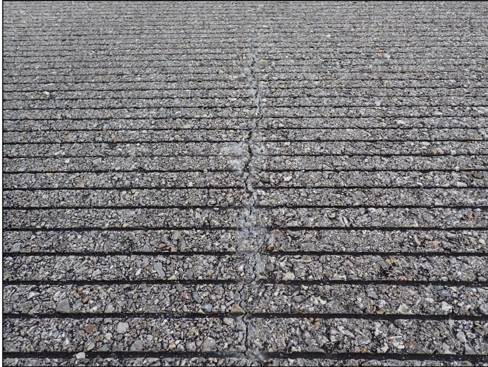
RW08-34-10: L&T Cracking
