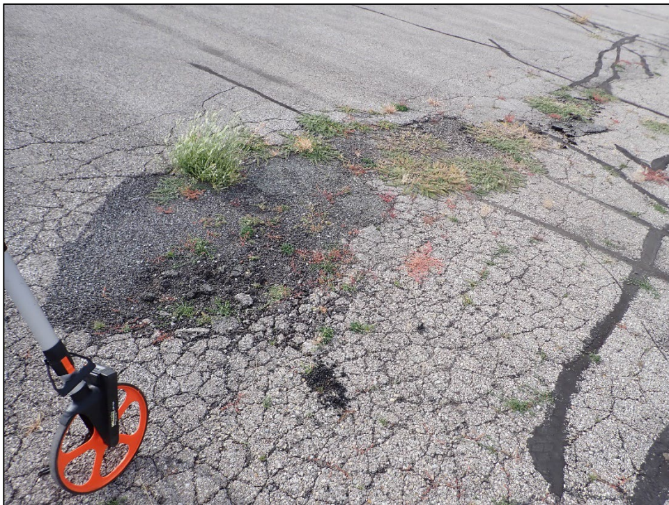
AP-03A-02: Alligator Cracking
