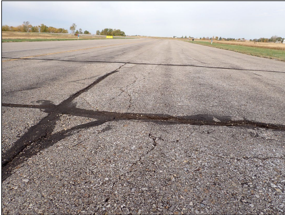
TW-07-03: L&T Cracking
