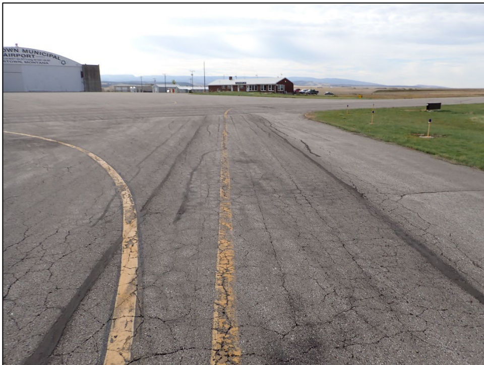
TW-88-01: Alligator Cracking
